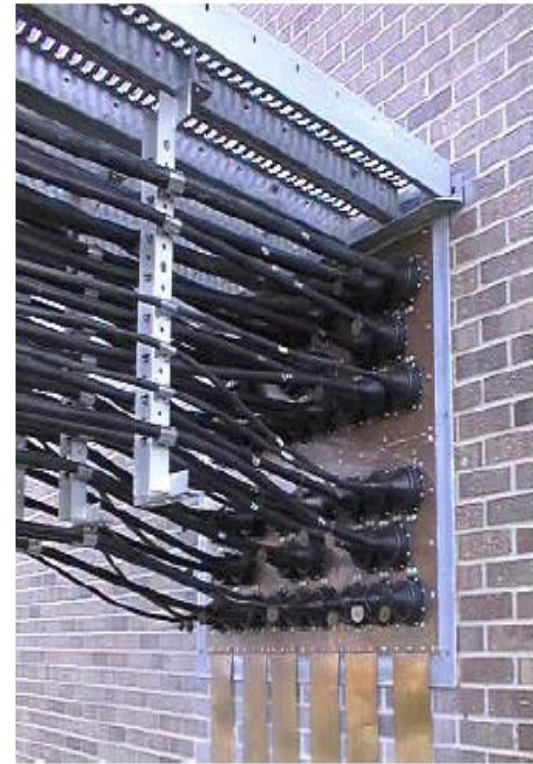
FIGURE 6-12 INTEGRATED CABLE ENTRY PORT WITH GROUND STRAPS
