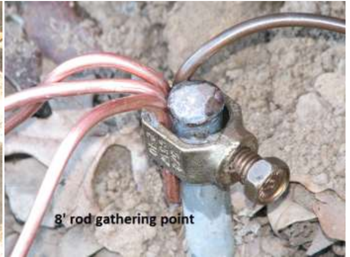
8' ground rod at base of tower, #1 awg wire
